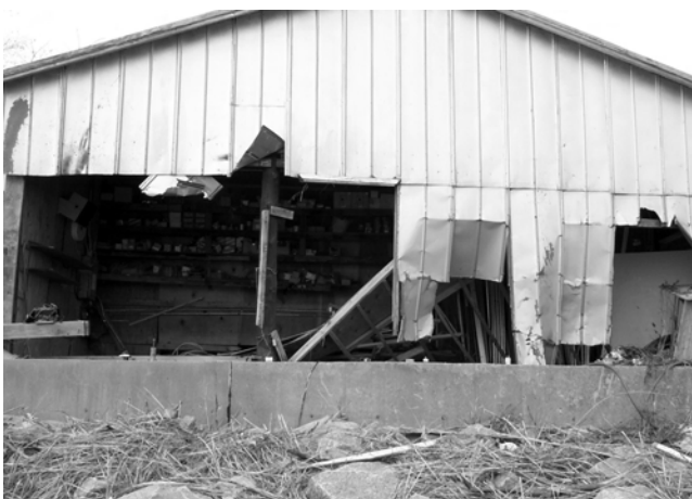
The electrical shop sustained severe damage.
