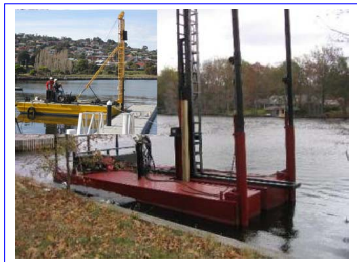
Figure 5.5 Small pile driving work barge (Source: ASD Pty Ltd., Marine Pile Drivers)
