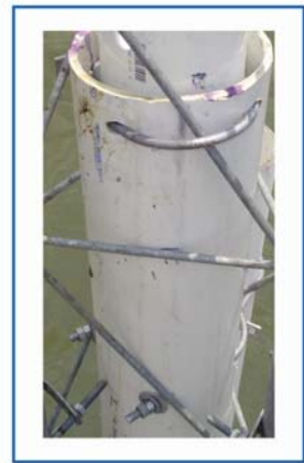
Figure 5.30 View of two U-bolts in a cross position.
