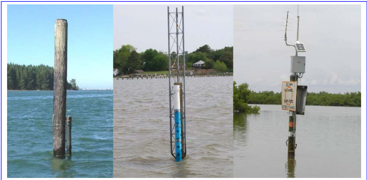
Figure 5.13 View of different pile platforms (Source: CBNERRVA, South Slough NERR, Rookery Bay)
